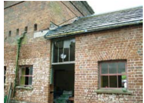
A section of lime mortar repointing and mould from leaking drain down pipe
