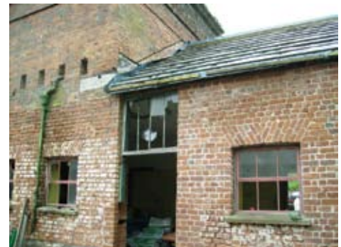
A section of lime mortar repointing and mould from leaking drain down pipe
