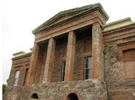
This photo shows exposed brickwork on ‘incomplete’ façade of Silverton Park Stables
