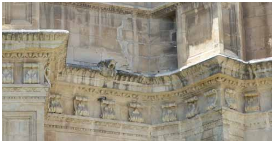
Figure 15. A view of the rear of the monastery showing the results of poor housekeeping and maintenance practices
