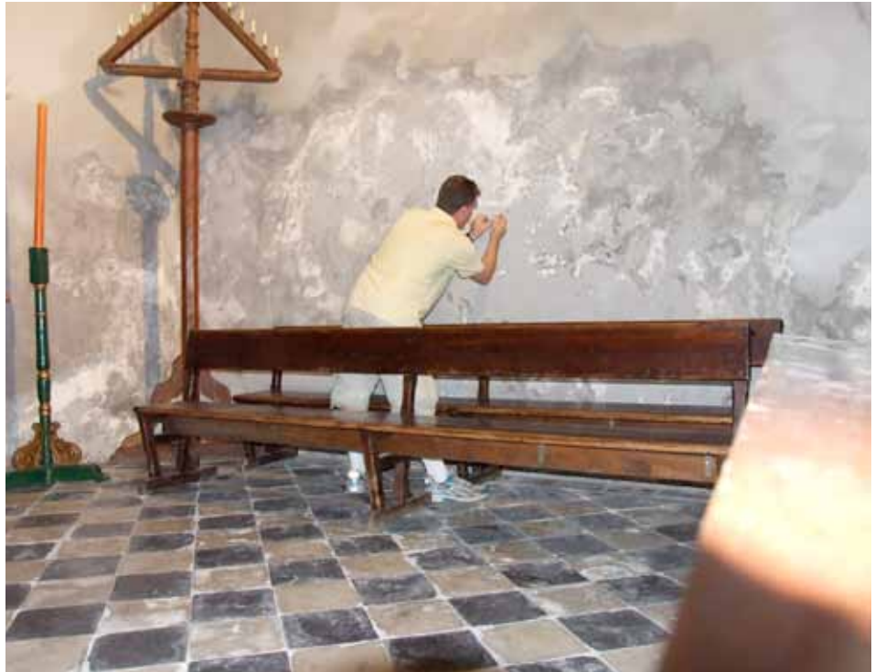
Figure 16. An example of penetrating damp
