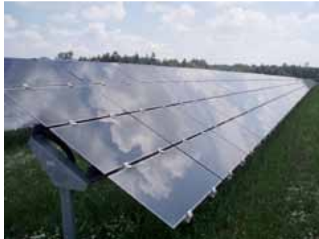
Long array four panels high
