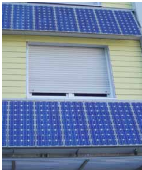
Apprentices Hostel With PV panels
