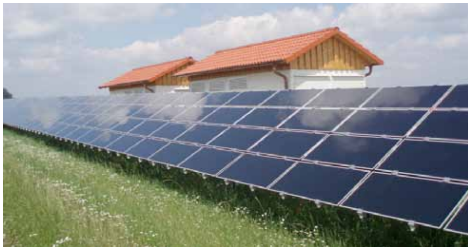
Panels and control buildings
