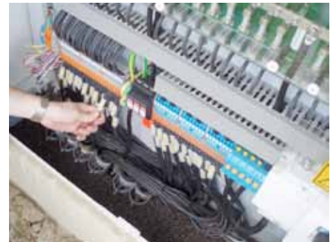
String monitoring unit under PV panels
