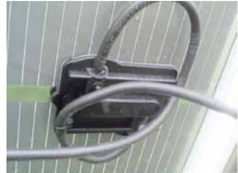
Cables (+ and -) at rear of a PV panel
