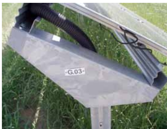
Support for PV panels
