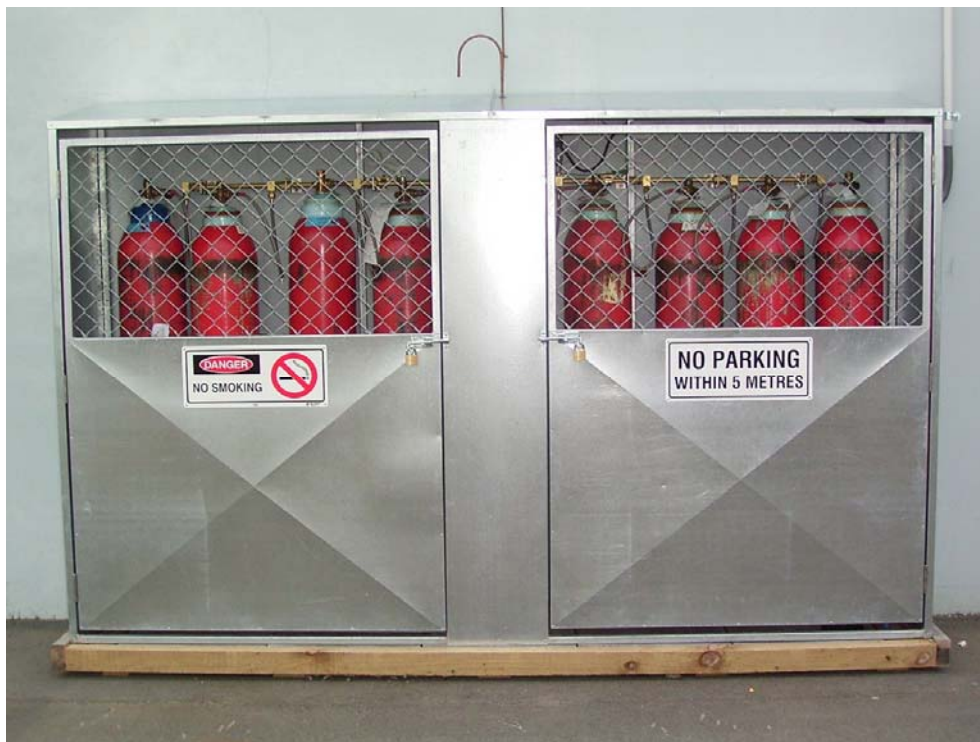
Hydrogen Storage Cage
