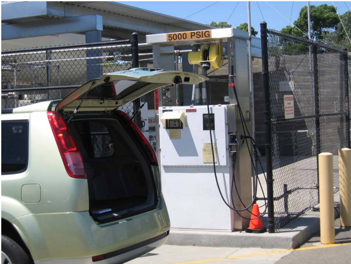
Hydrogen Refuelling Station
