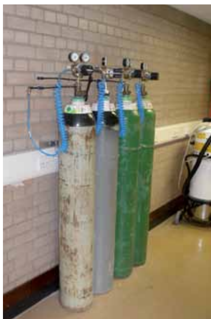
Manifold storage of inert gas for use in RM machine for metal parts at Material Solutions, the University of Birmingham
