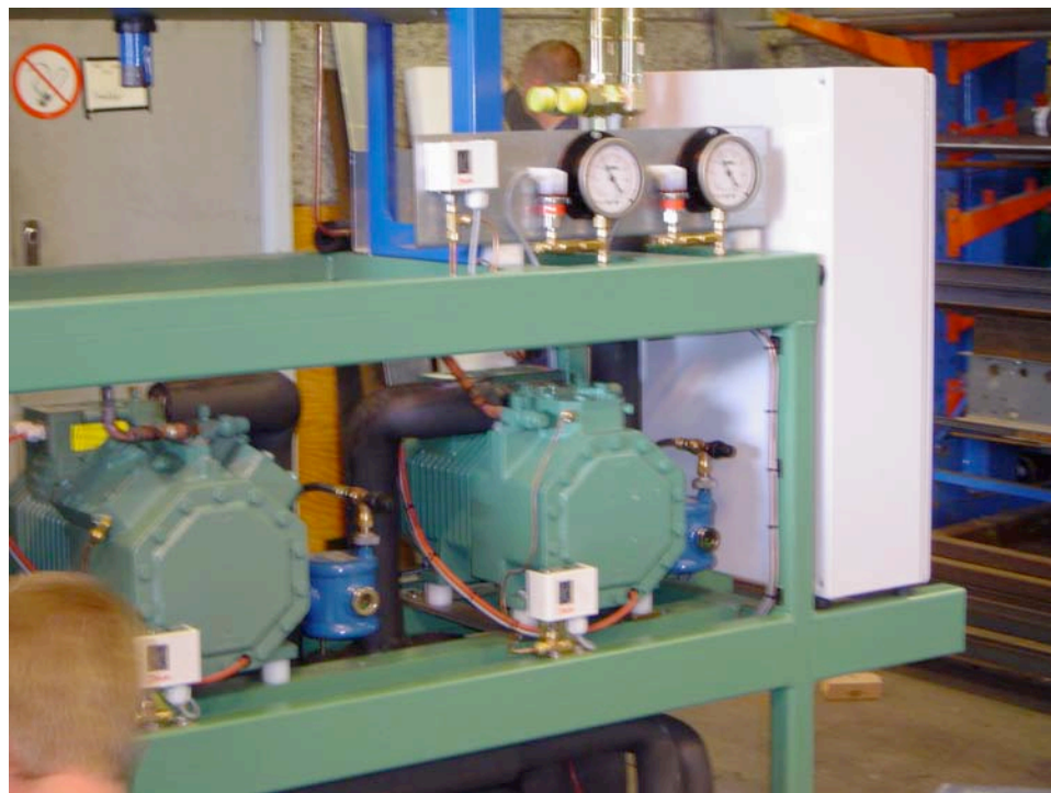
York CO 2 Refrigeration package
