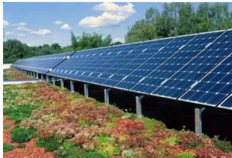
Photovoltaic integrated design - Germany
