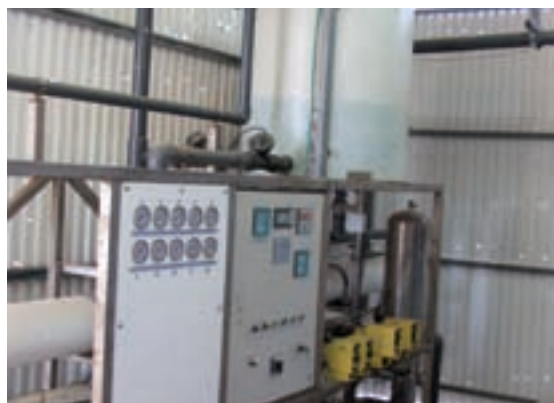
Reverse osmosis equipment
