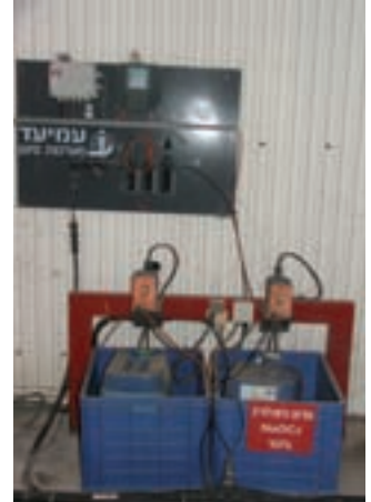
Sodium hyperchlorite injection system
