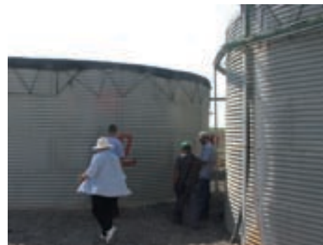
Mixing tanks dam water and waste water from the nursery
