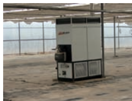
Production area ready for planting showing gas heating system
