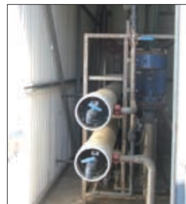
Reverse osmosis equipment
