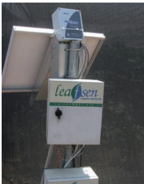
Leaf-Sen controller box with solar cell charging unit
