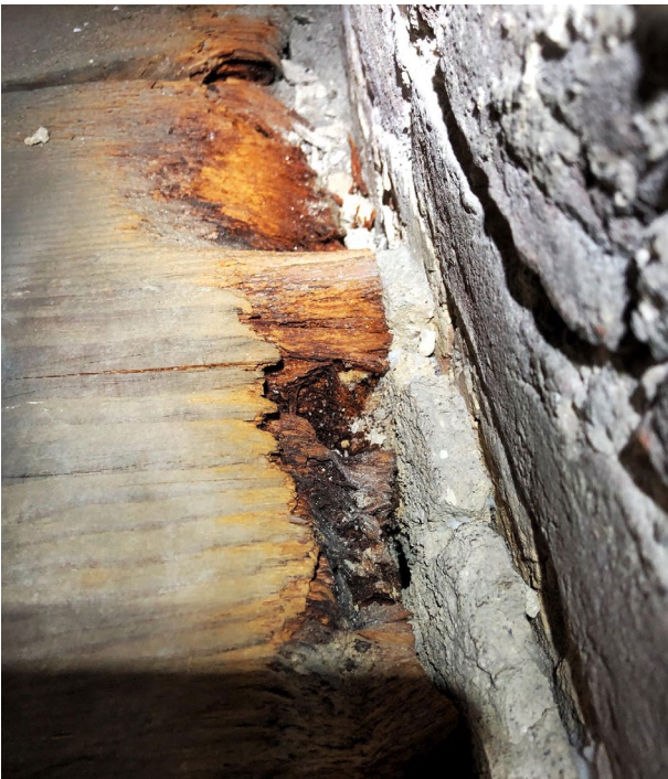
Figure 7. Degradation of timber found beneath piles of debris and detritus in the Portuguese Synagogue.
