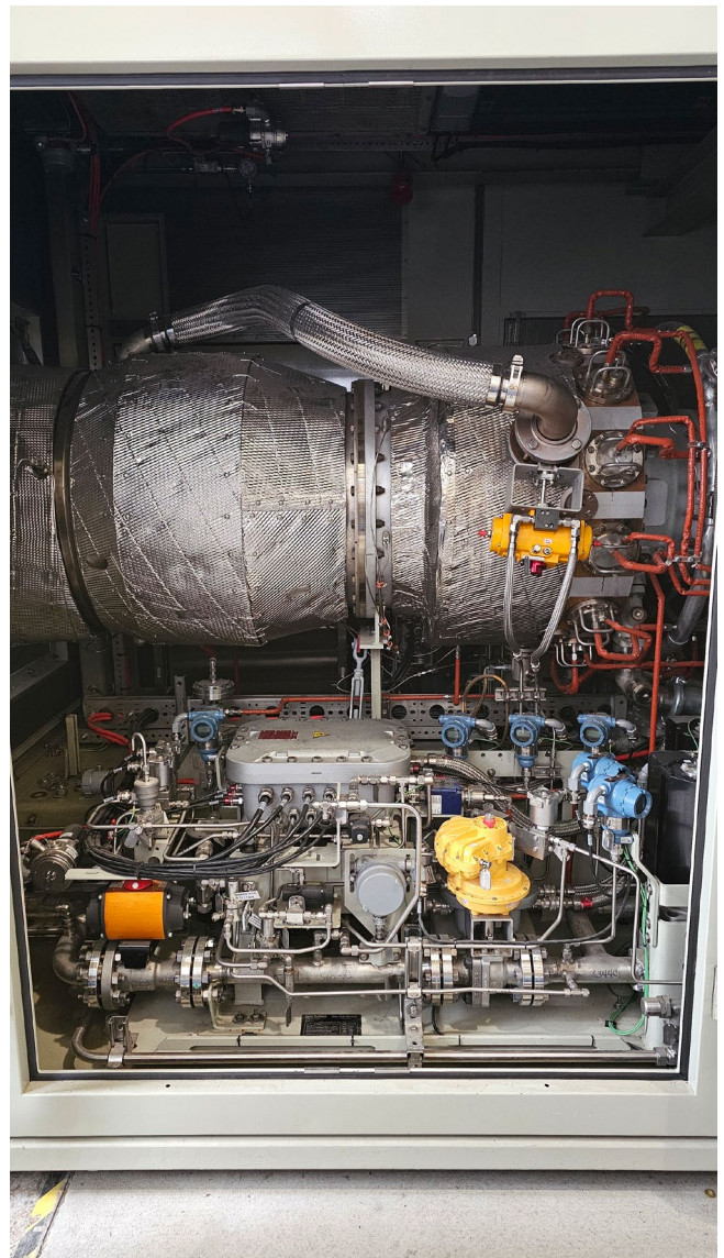
Figure 15: Image of the CSU hydrogen & natural gas generator. It can be used to power the entire campus, with a combination of hydrogen and natural gas.
