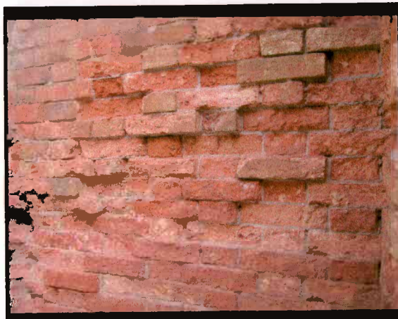
Decaying brickwork Venice
