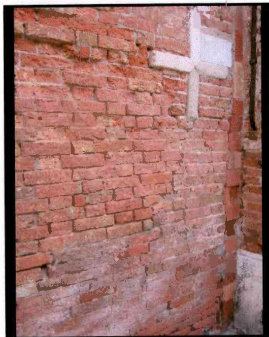
Salt damaged brickwork Venice
