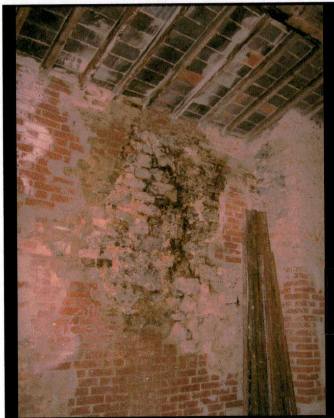
Water Damage. Villa Demidoff. Florence
