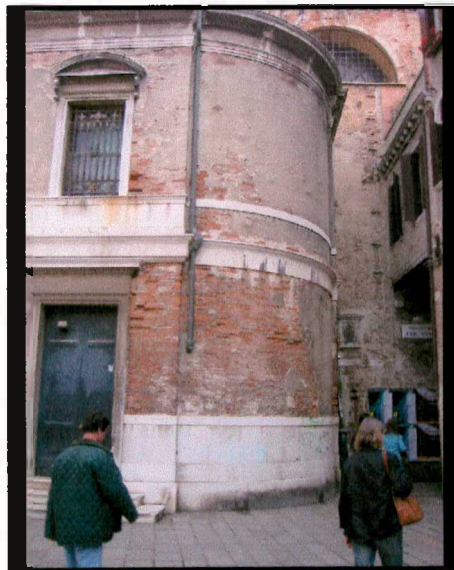
Crumbling brickwork. Venice.
