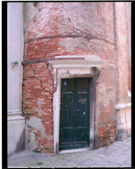
Crumbling brickwork. Venice
