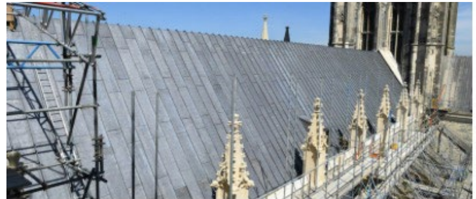
View from western tower scaffold to the 235-foot-high Bell Harry Tower. Approximately 56 metric tonnes of lead had been taken off the roof, recycled and re-laid. (Credit TH) .
