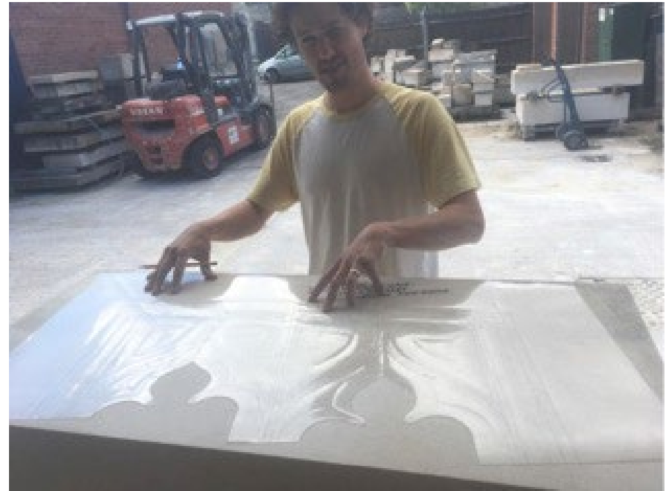
James Bayliss applying templates for an open tracery parapet merlot, using French Lepine limestone due to the tall bed height requirements over 600mm.
