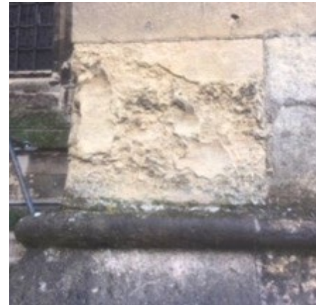
Decayed local Dalton stone showing considerable surface deterioration, accelerated due to the action of atmospheric pollutants (TH)
