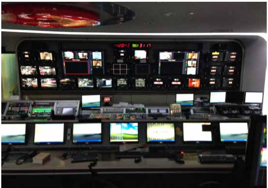
SMG TV Control Room
