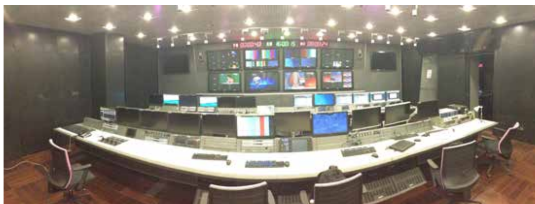
CCTV Control Room
