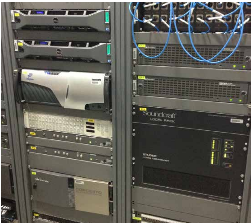
SMG Dragon Server/Router rack
