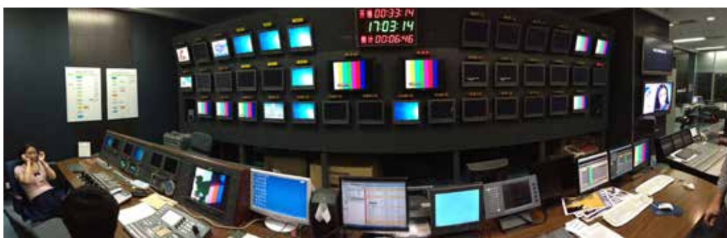
Nanjing Control Room wide shot
