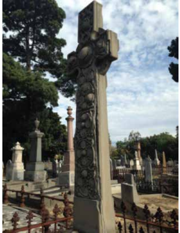
Badly deteriorated sandstone monument Melbourne General Cemetery. Can stone this badly damaged be recovered by conservation?
