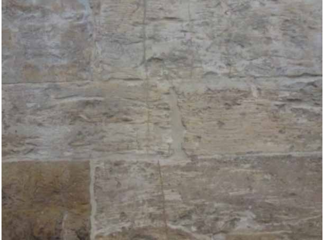
Parma Cathedral wall, losses in stone repaired with almost invisible mortar repairs
