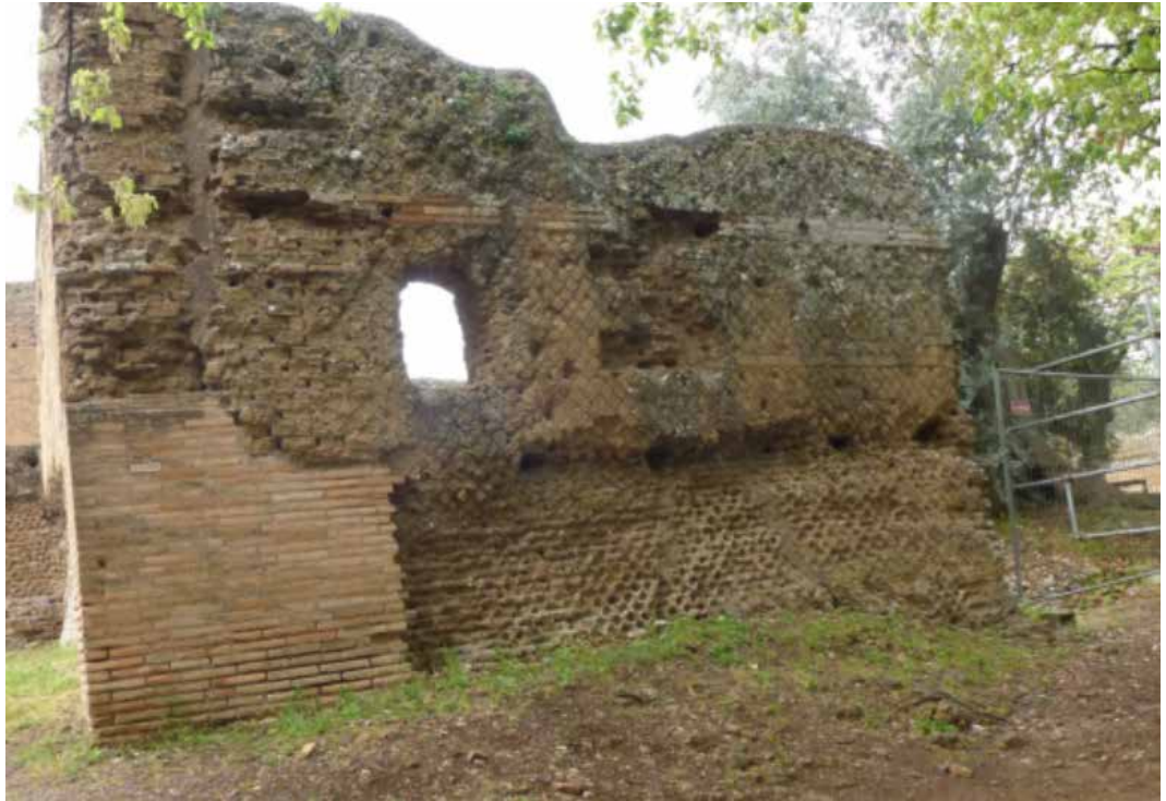
Wall at Hadrian's Villa with losses at the base caused by salts
