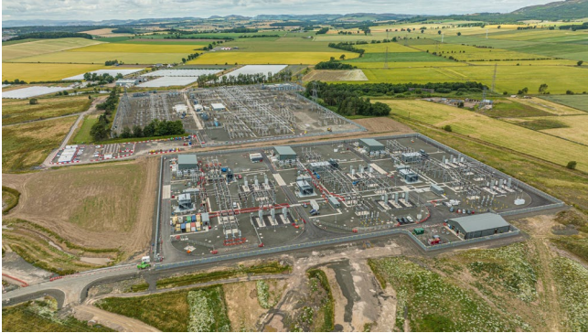
Figure 9. Tealing Substation in the foreground 19kms from landfall serviced by 3 underground transmission cables, measuring 45,000 square meters in area.
