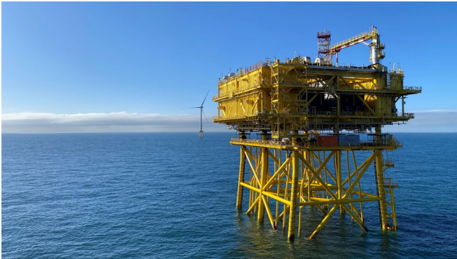
Figure 14. Completed Offshore Substation
