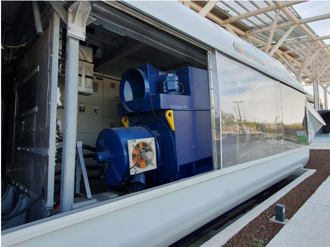
Figure 21. A nacelle used for training purposes (ground mounted) with Perspex windows to allow for easy access to undertake training activities
