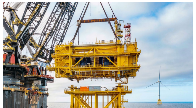
Figure 13. Installation of the Offshore Substation on the jacket foundations, completed wind turbine in the background.
